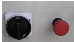
Fig. 3. Disconnect switch and emergency stop button (red)
